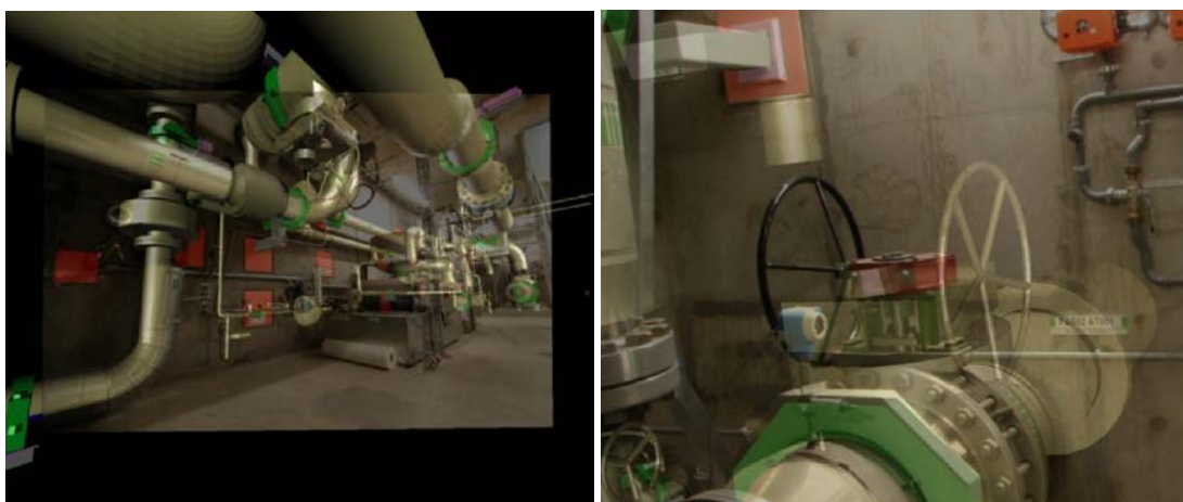
Figure 1. AR can be used for discrepancy analysis in industrial facilities. The images show still frames overlaid with CAD information. Note how the valve on the right hand side was mounted on the left side rather than on the right side as in the model.
